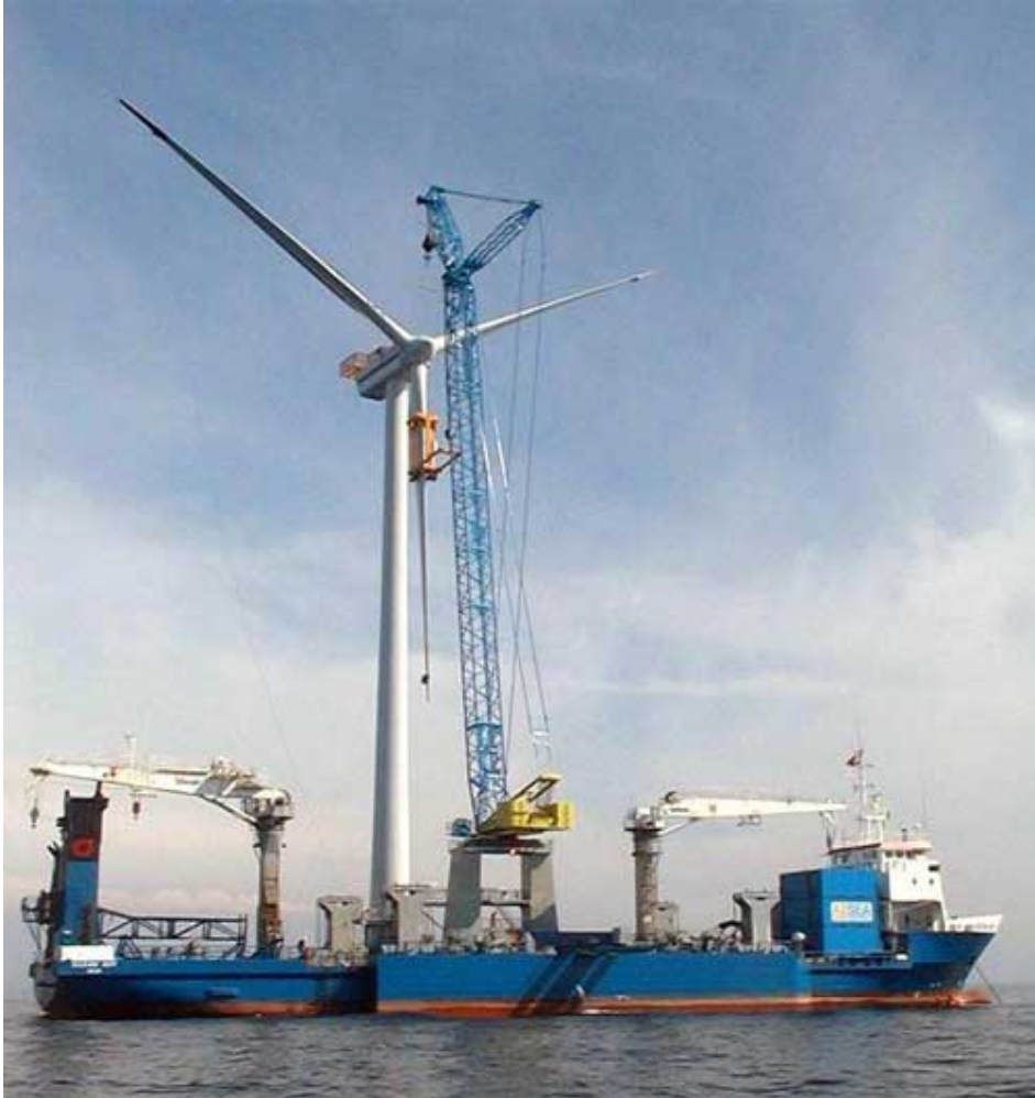
Fig. 4.9: Blade being mounted; the nacelle, hub and two blades have already been assembled onshore
